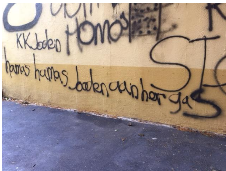
Graffiti in a tunnel: "Hamas Hamas Jews to the Gaz"
